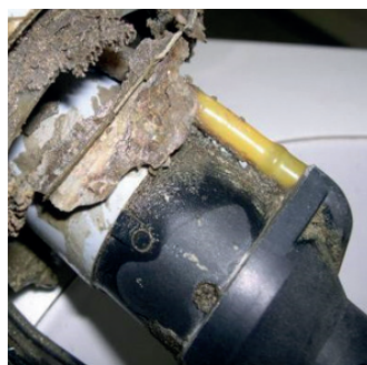
Deposits on module 2
